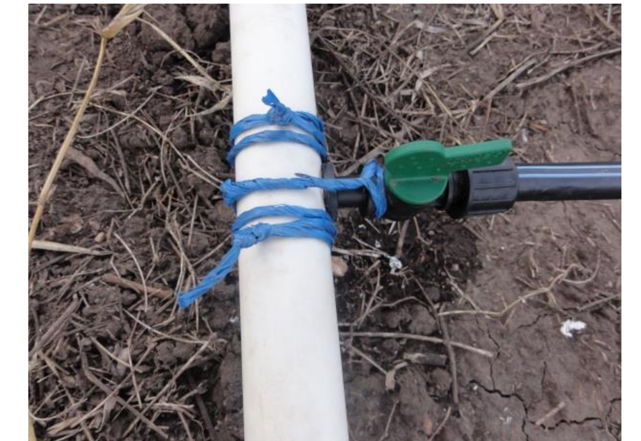
Figure 3. Drip line water flow controllers
